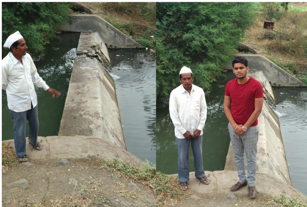
Photo-3- Under repairing of check dam situated on nala of Ghatangri watershed
