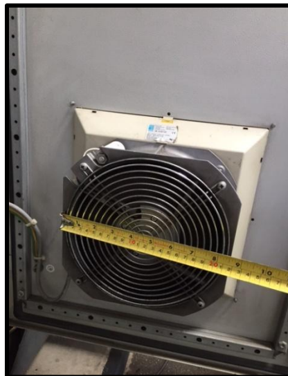
Figure 10: Measurement of the diameter of fan installed on the VFD panel.
