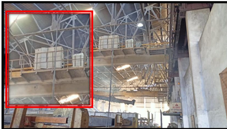
Figure 2: The IB – 55 grade VFD panel on the heavy duty “Electromech” crane.
