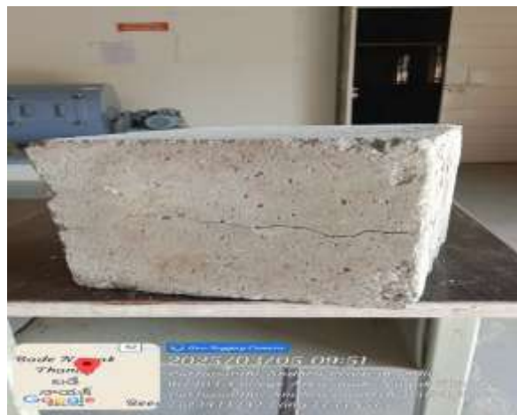
Cracked concrete brick
