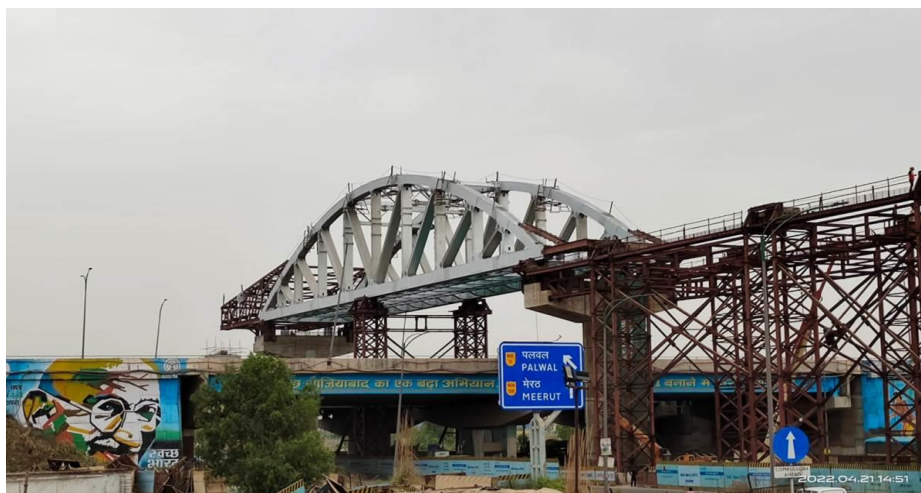
Fig 1: Design of Long Span under Construction Project for the Delhi–Meerut RRTS Metro rail Bridge Structure
