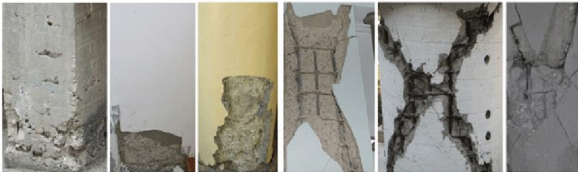
Fig 1: Spalling of Concrete in different Types of Structures
