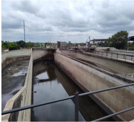
Waste water treatment plant
