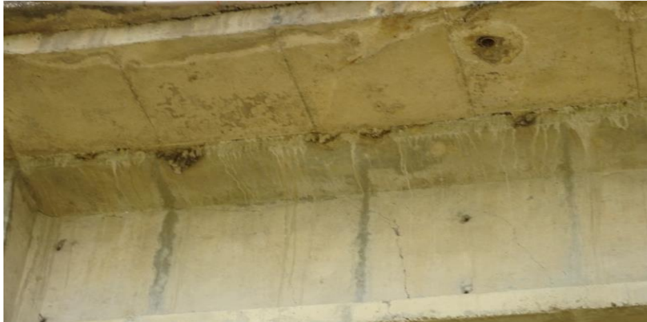
Figure 1. Longitudinal Crack in web of Beam from bottom to top face
