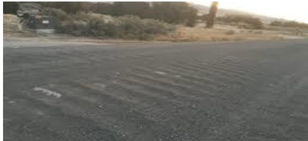
Figure h) corrugation cracking
