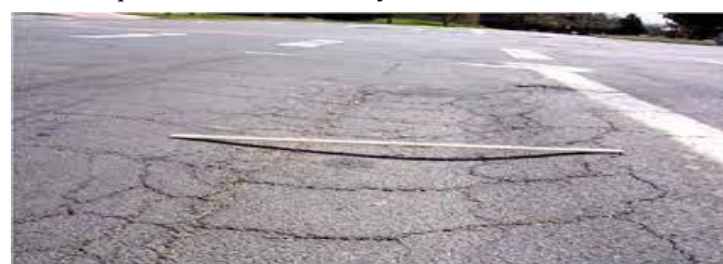
Figure e) rutting
