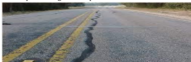
Figure a) longitudinal cracking
