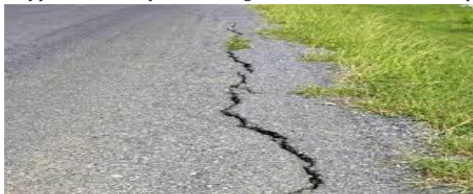
Figure d) edge cracking
