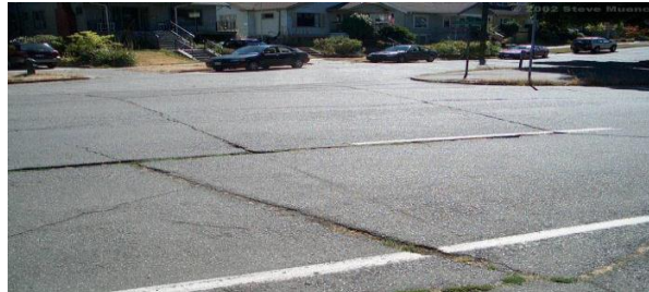
Figure g) reflection cracking
