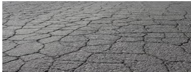
Figure b) fatigue cracking
