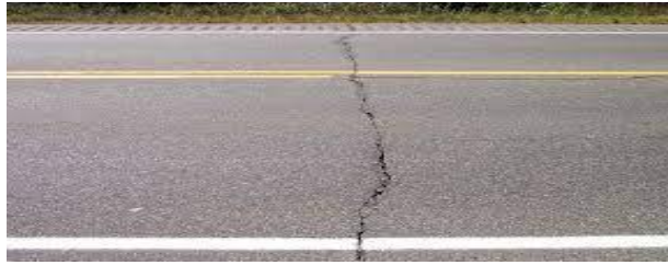
Figure f) transverse cracking
