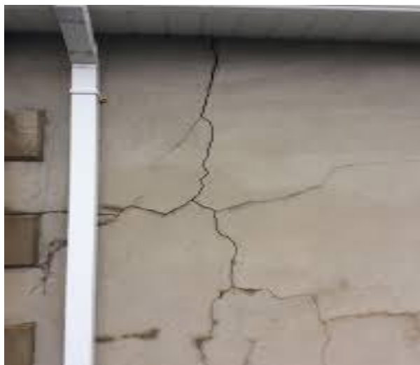
Cracks Forming Due to more absorption of water from concrete
