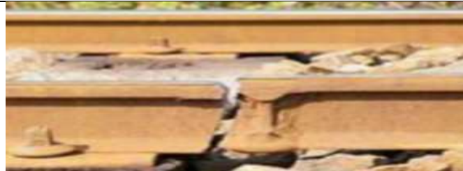
Figure 1. Railway Track Crack
